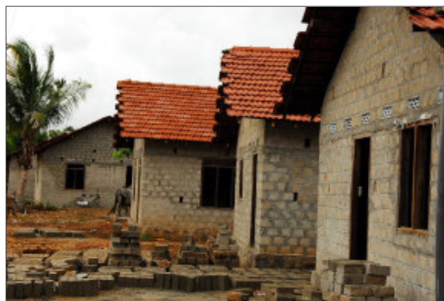
Houses being constructed through an American Red Cross owner-driven housing initiative in Sri Lanka.
