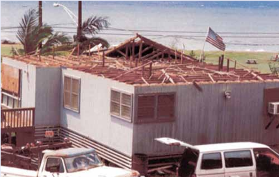
Figure 2-6. A common site on Kauai after Hurricane Iniki. Many roofs were blown off due to a lack of proper connection. Photo courtesy of Department of Commerce and Consumer Affairs Insurance Division.
