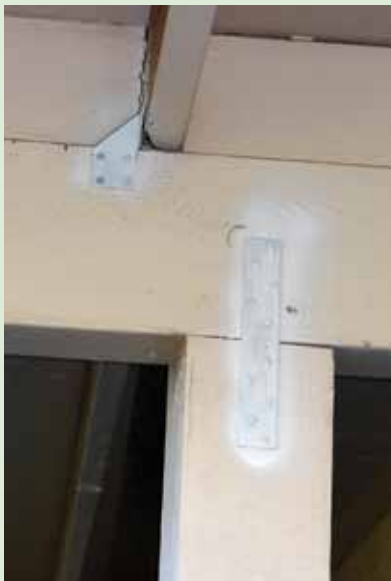
Figure 4-5. In this retrofit example, a hurricane clip attaches the roof structure to a horizontal ridge beam, which is in turn attached to the vertical post with a metal strap. This is an attempt to tie the load from the roof to the foundation, or create the complete load path connection. Note that these clips and straps are in the process of being painted. Photo courtesy of Hurricane Protection Services.
