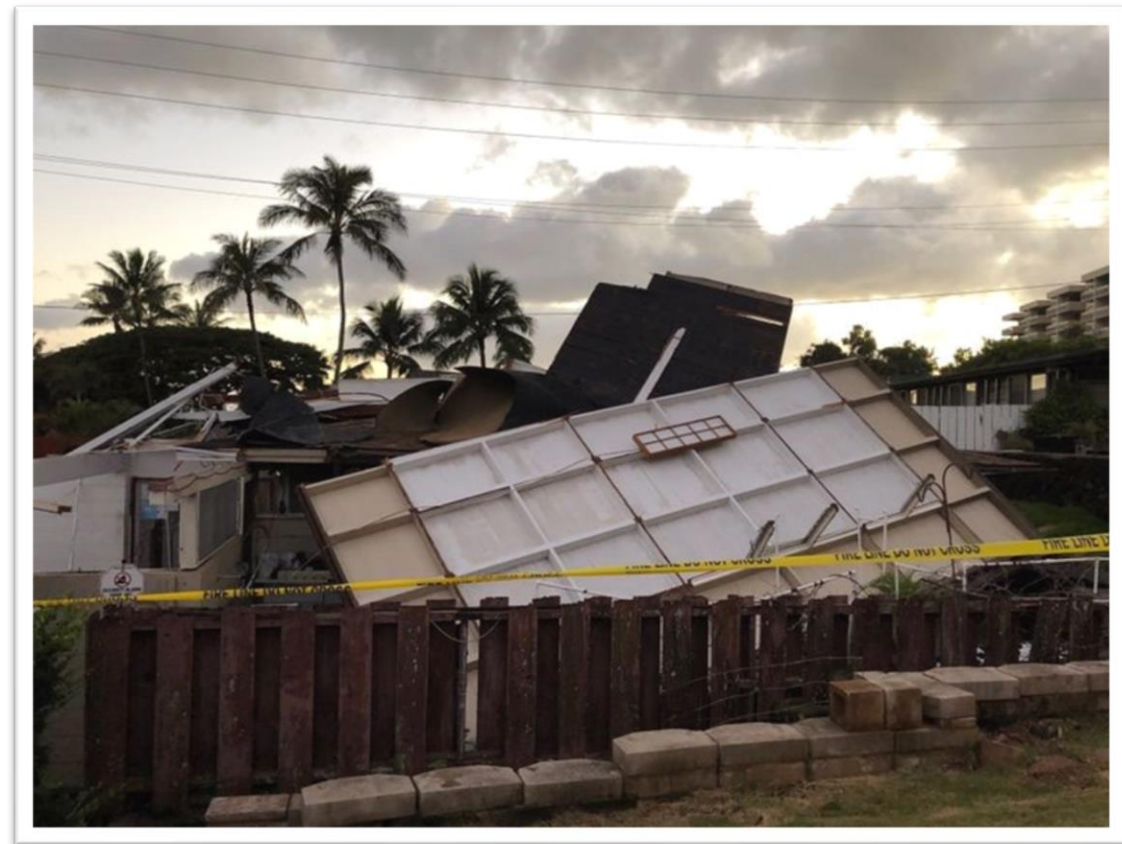
Roof blown off in Kahala earlier this year
